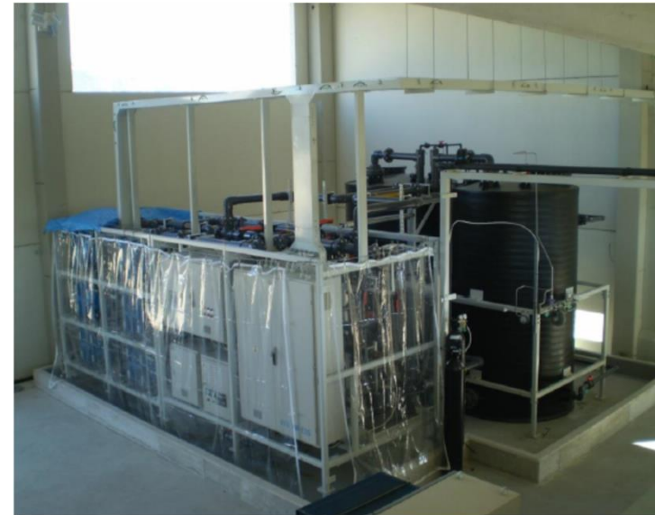
S- Redox Battery 50 kW x 4 hours
